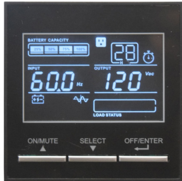
HMI showing key UPS parameters
