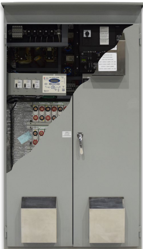
NEMA 3R charger fitted with double doors and rain hoods over vents. Integrated battery rack w/ 20 yr. VRLA batteries.
