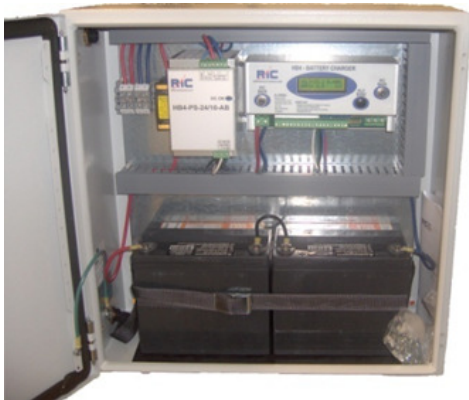
Integrated Battery Racks
